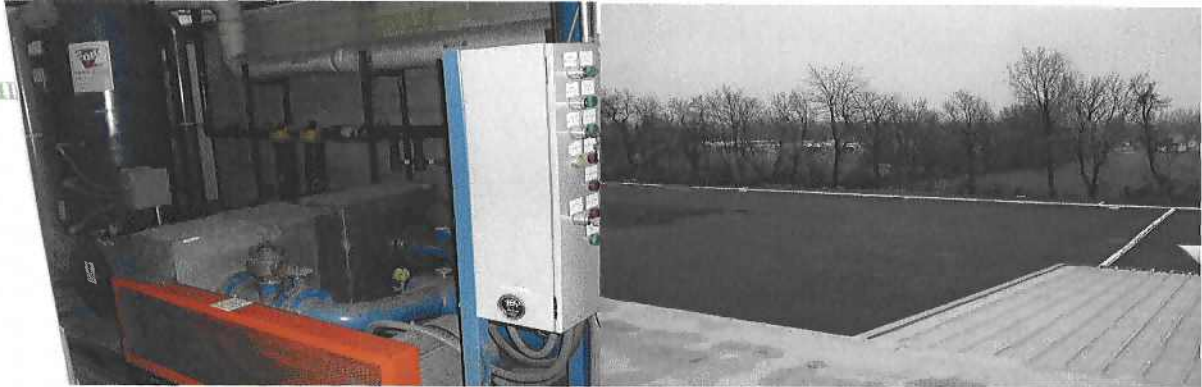
Figures 1 & 2 – SVE vacuum blower unit and southern piping connection system at SEA Ohio site.
