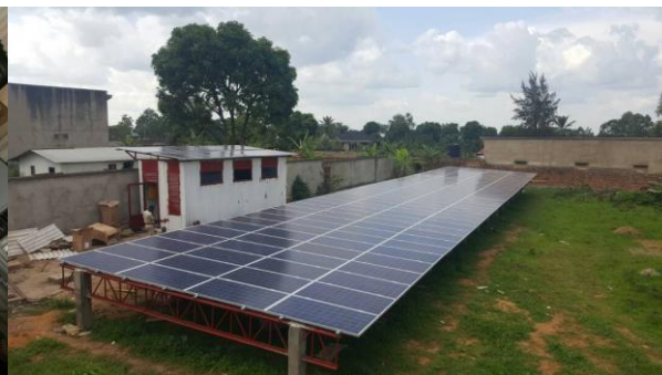
Figure 3. 55 kW PV Array (Photo by Bidong, E.)
