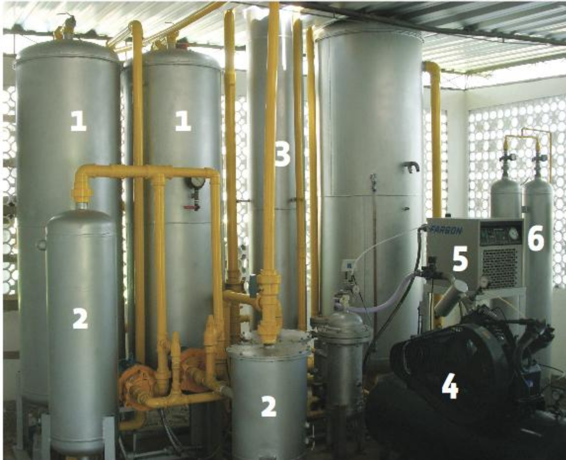
Figure 3. Biogas Purification System
