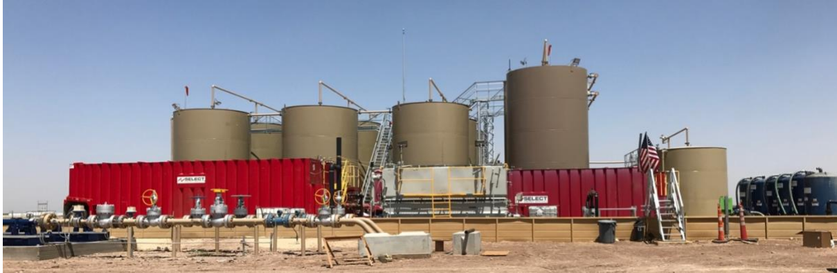
Figure 4. Chiltepin Recycling Plant, Pecos, Texas. Foreground is Select Energy Services Treatment Interventions from left to right, settling tanks, gas flotation unit, and filtration. Background from left to right tank battery, gun barrels and additional tank associated with disposal at SWD.
