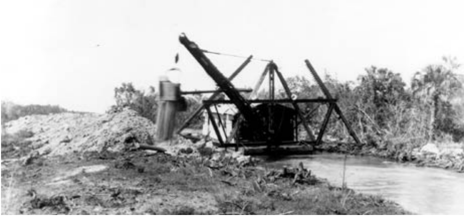
Figure 4. A Bay-City dredge, circa 1927, excavates sand and limestone to create the Tamiami Trail. Retrieved February 24, 2007 from Collier County Museums. (2001). Tamiami Trail: History and Photos . http://www.colliermuseum.com/history/tamiami_pic3.htm .
