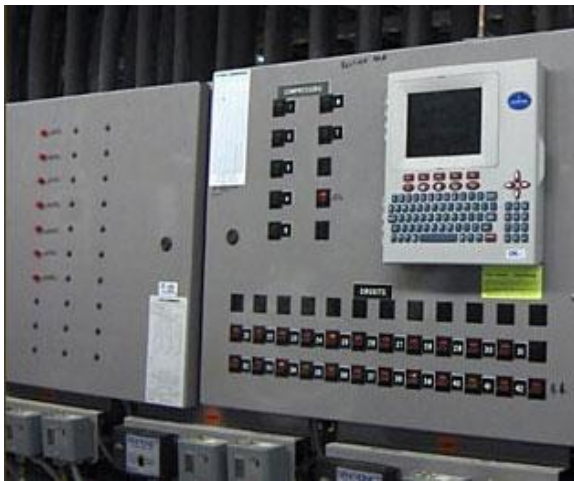
Figure 26. Example of an EMS. Source: http://www.stonesriverelectric.com/energy-solutions/energy-management.html
