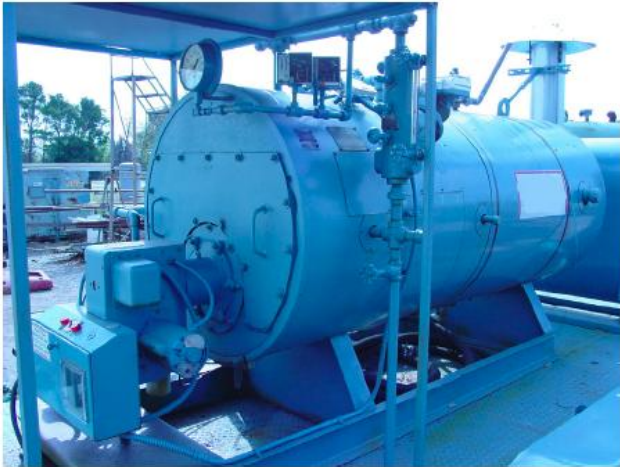
Large residential steam boiler—oil fired
