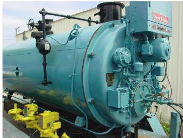
Residential hot water boiler—gas fired
