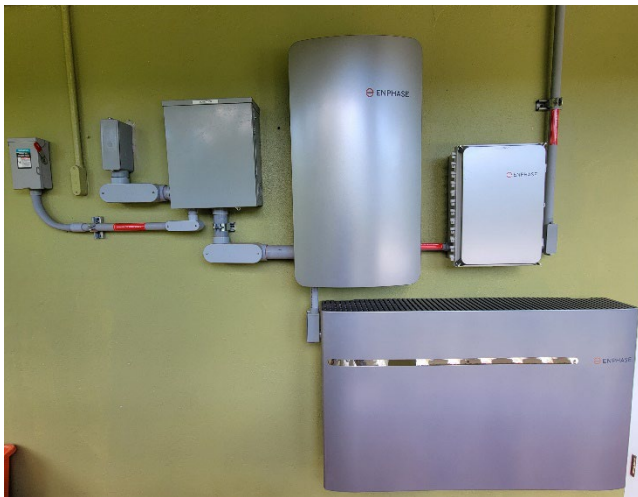
System controls and battery for the solar and storage system installed at a house. Photo courtesy of EDF.
