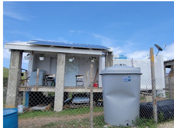
Some homes, like the one above, required structural reinforcements to accommodate solar panels on the roof. Photo courtesy of EDF.
