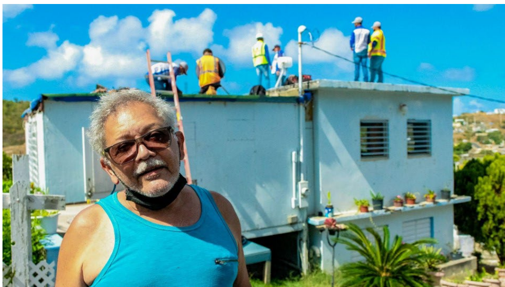
A project participant during the installation of solar panels on his roof. Photo courtesy of EDF.
