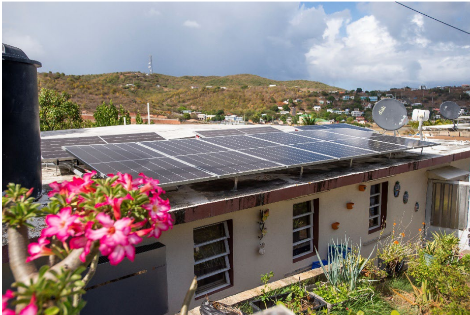
The larger installation configuration can power the basic needs of a household with two or more people. Photo courtesy of EDF.
