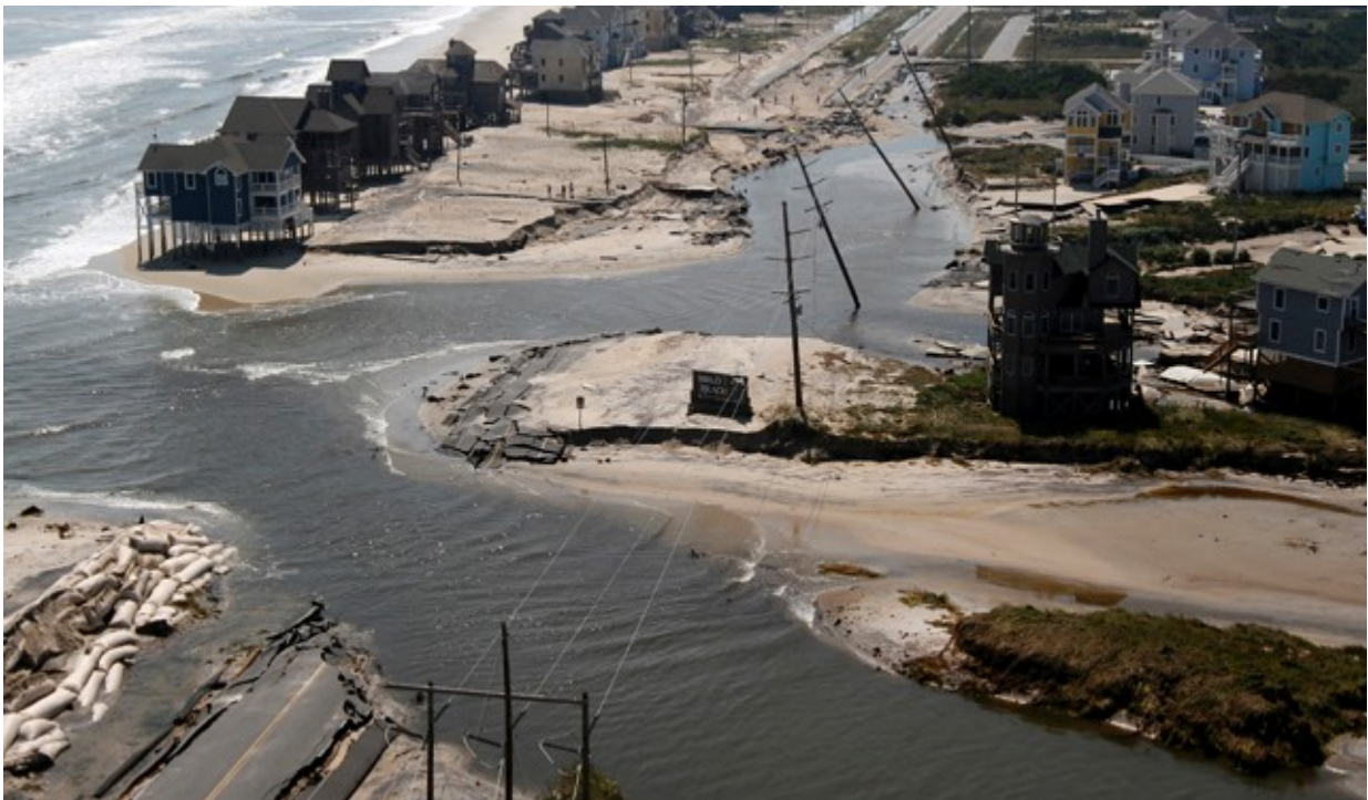
Figure 9. One of two breaches of NC 12 after Hurricane Irene in 2011 north of Rodanthe, NC (Associated Press, 2012).
