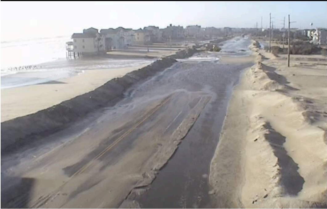
Figure 2. Sand and water on NC 12 north of Rodanthe, NC on March 9, 2013 (NCDOT, 2013a)
