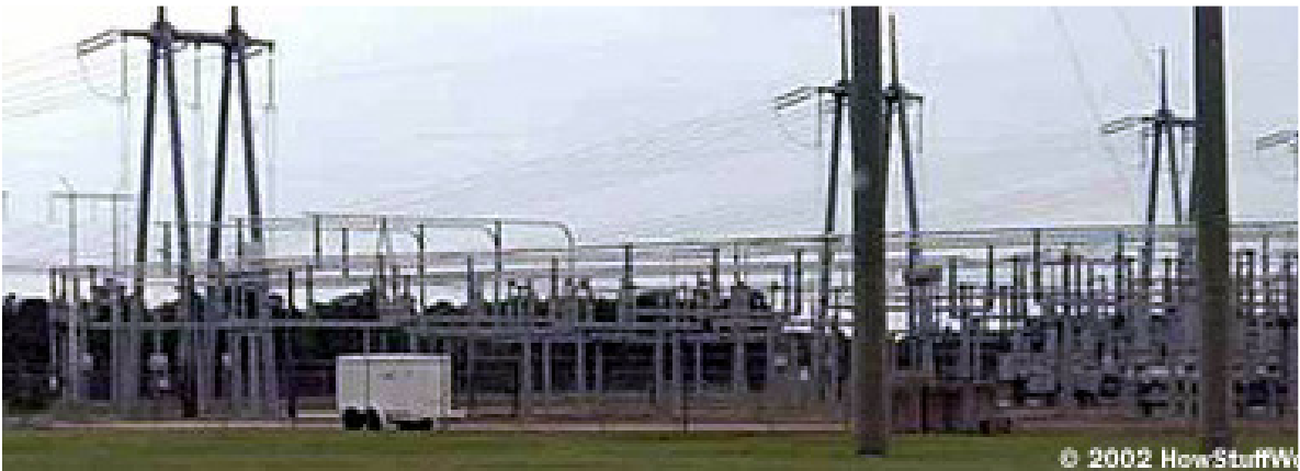
An electricity substation
