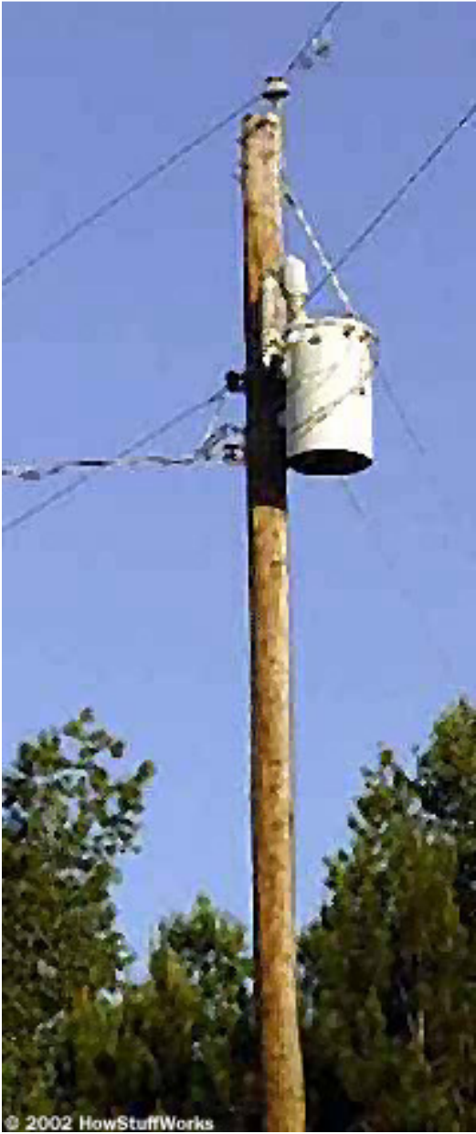
A transformer drum
