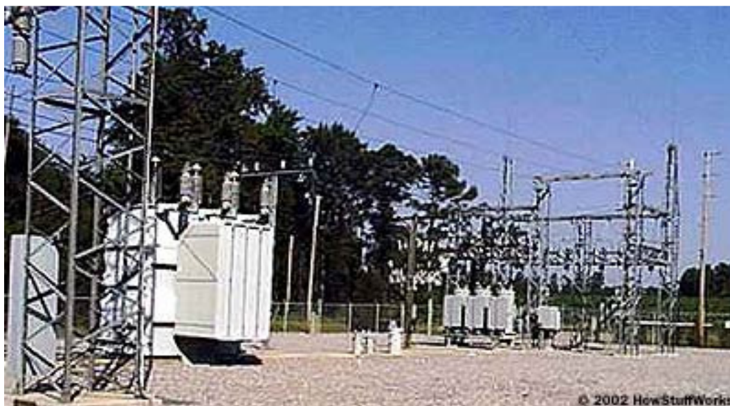
An electricity substation
