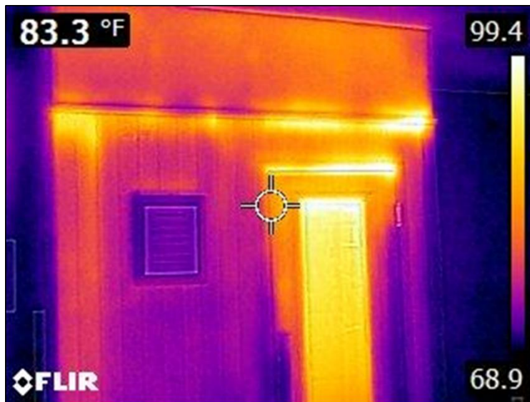
Figure 18. Infrared Image of Property 3 Sauna
