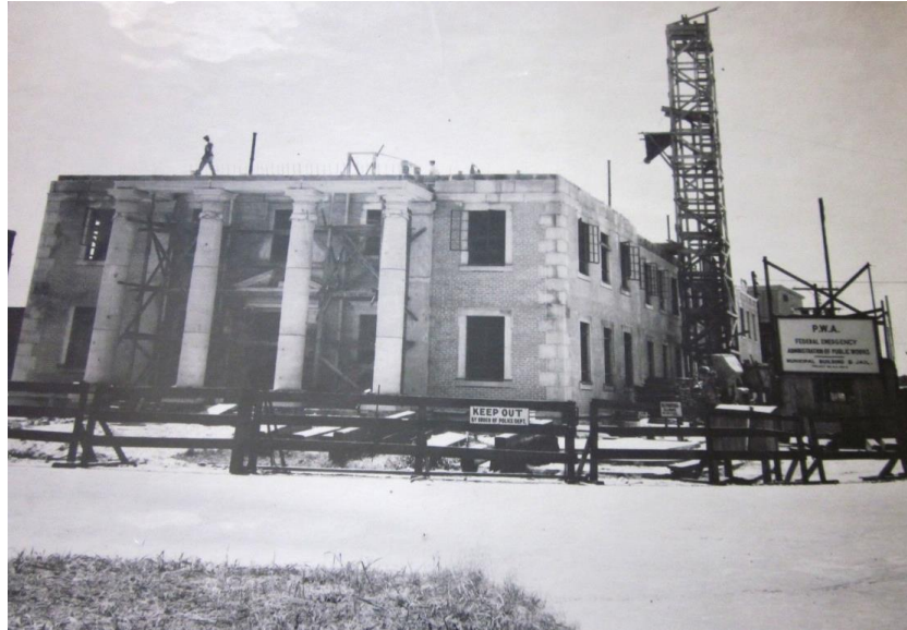
Figure 17: Construction of Selma municipal building and jail as PWA project during 1937. The building directly behind the construction site is the newly-completed Negro Community Center, also a PWA project. Courtesy Billy Rosenberg Photograph Collection, Temple Mishkan Israel.
