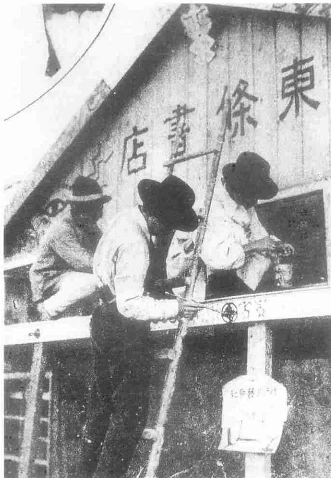
FIGURE 4. Barrack Decoration Company members shown on a ladder painting the facade of the Tōjō Bookstore, Jimbochō. Reproduced in a montage of photographs entitled 'Fukkō tojō teito 1' (The Imperial Capital in the Process of Rebuilding 1), Asahigraph 1:1, 14 November 1923, p. 4.
