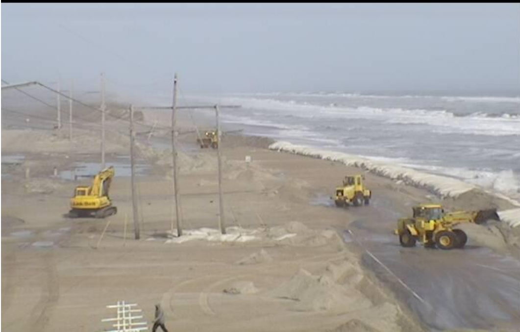
Figure 3. NCDOT clearing sand from NC 12 north of Rodanthe, NC on March 11, 2013 (NCDOT, 2013a).
