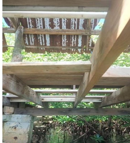
Figure 5 Papago boathouse roof, holes in the roof led to a range of lidar return values.
