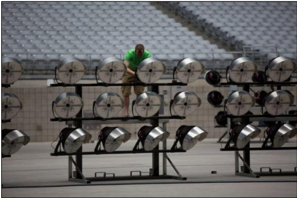
Figure 8: LED Installation (Ringle, 2015)
