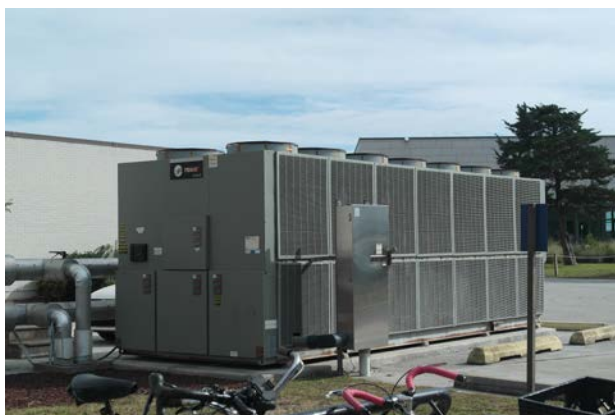
Figure 31. A chiller unit is shared between Bookhout Laboratory and Library / Auditorium. Uneven cooling load may be negatively impacting the Library.
