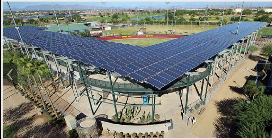
Figure 36. PV panels installed at the top of the stadium seats of a baseball field in one of ASU campuses.
