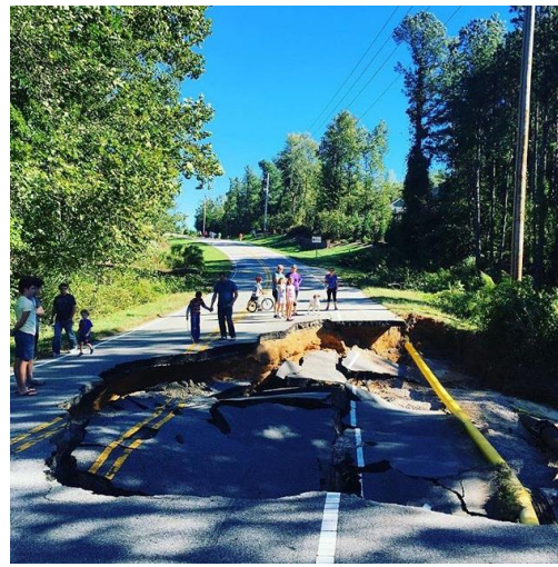
Fig. 2. Road washed out in Wake Forest, NC after Hurricane Matthew, October 2016. Photo by Ashlie White.
